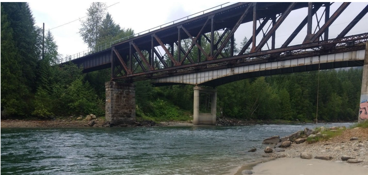
Figure E-26. Highway 3A and Railway Bridges over the Slocan River from left bank looking upstream. Photo: Midwest Survey July 4, 2019.
