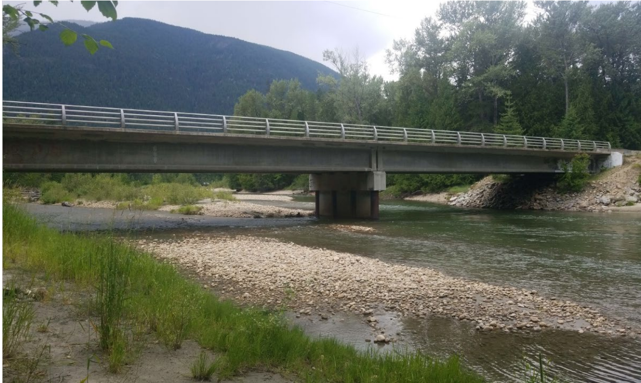
Figure E-19. Little Slocan Bridge over the Little Slocan River from right bank looking upstream. Photo: Midwest Survey July 8, 2019.
