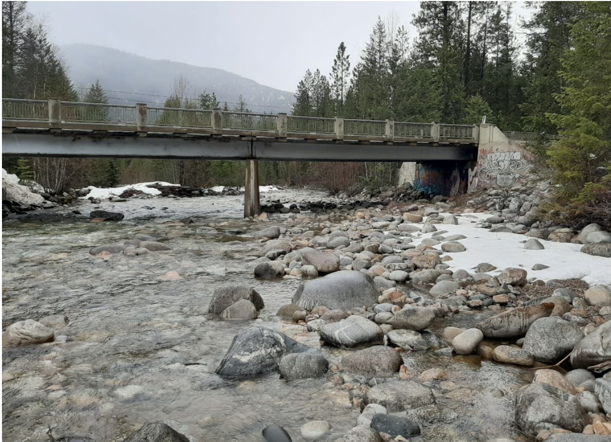
Figure E-11. Highway 6 bridge over Lemon Creek standing in the channel looking upstream. Photo: Brian Cutts March 29, 2020.
