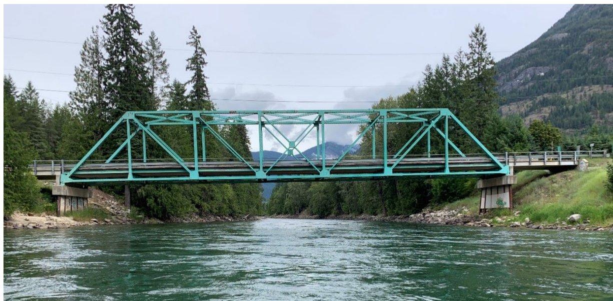
Figure E-23. Slocan Park Bridge over the Slocan River from the channel looking upstream. Photo: Midwest Survey July 8, 2019.
