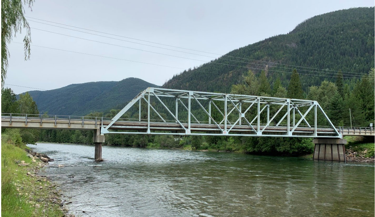
Figure E-20. Passmore Bridge over the Slocan River from left bank looking downstream. Photo: Midwest Survey July 8, 2019.
