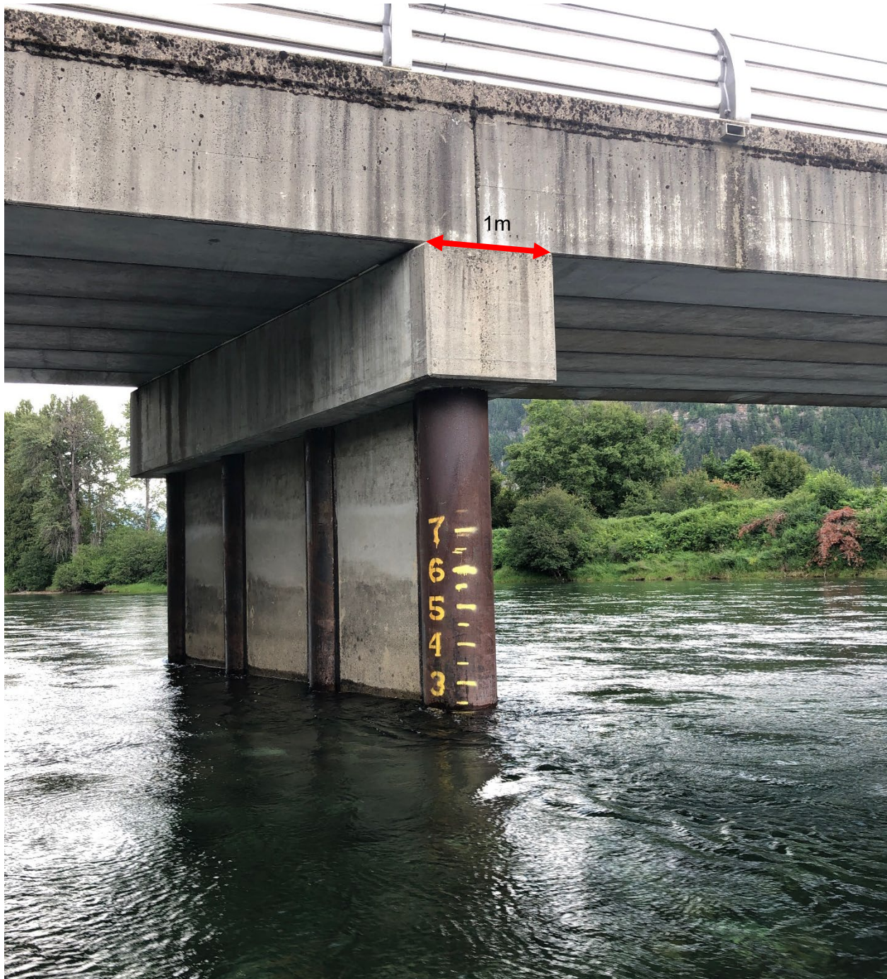
Figure E-9. Slocan City Bridge over the Slocan River looking at pier. Photo: Midwest Survey July 8, 2019.
