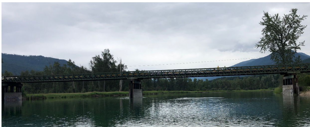
Figure E-17. Perry Bridge over the Slocan River looking upstream. Photo: Midwest Survey July 15, 2019.
