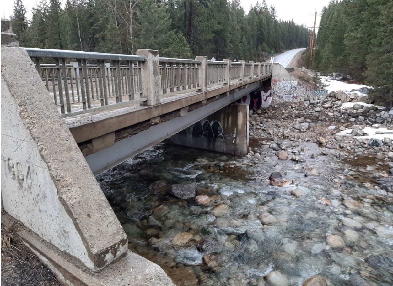
Figure E-10. Highway 6 bridge over Lemon Creek standing on the left abutment looking across. Photo: Brian Cutts March 29, 2020.
