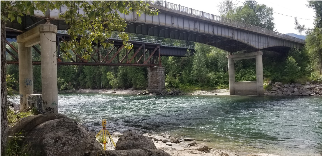
Figure E-25. Highway 3A and Railway Bridges over the Slocan River from left bank looking downstream. Photo: Midwest Survey July 12, 2019.
