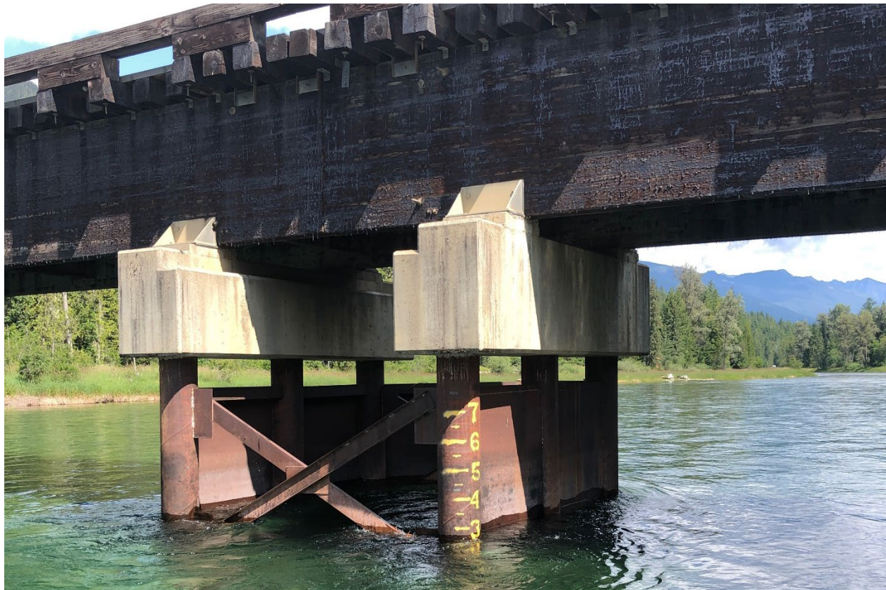
Figure E-15. Logging Road Bridge over the Slocan River looking at pier. Photo: Midwest Survey July 8, 2019.
