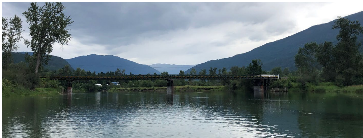
Figure E-16. Perry Bridge over the Slocan River looking downstream. Photo: Midwest Survey July 15, 2019.
