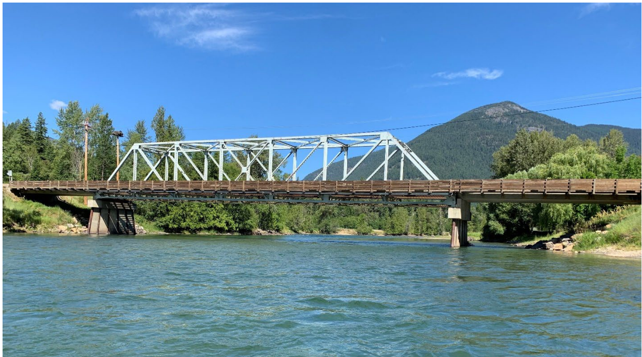
Figure E-21. Passmore Bridge over the Slocan River from the channel looking upstream. Photo: Midwest Survey July 8, 2019.
