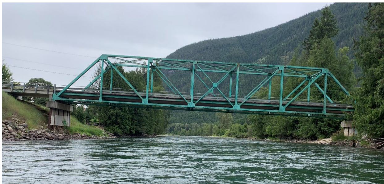
Figure E-22. Slocan Park Bridge over the Slocan River from the channel looking downstream. Photo: Midwest Survey July 8, 2019.
