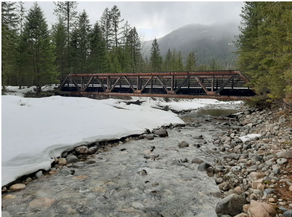
Figure E-12. Slocan Valley Rail Trail Bridge over Lemon Creek. Photo taken standing on right bank looking downstream. Photo: Brian Cutts March 29, 2020.
