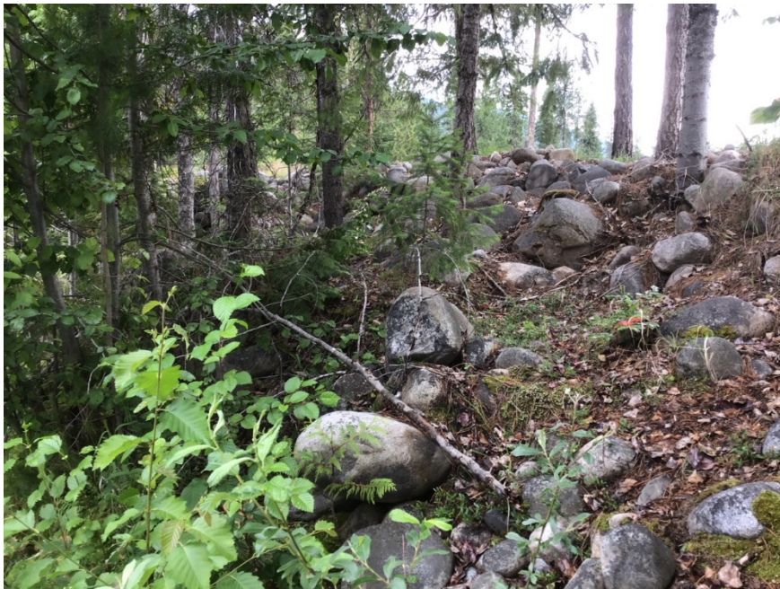
Photo 12. Lemon Creek rock protection on right bank 200 m west of Highway 6. Photo: BGC, July 2, 2019.
