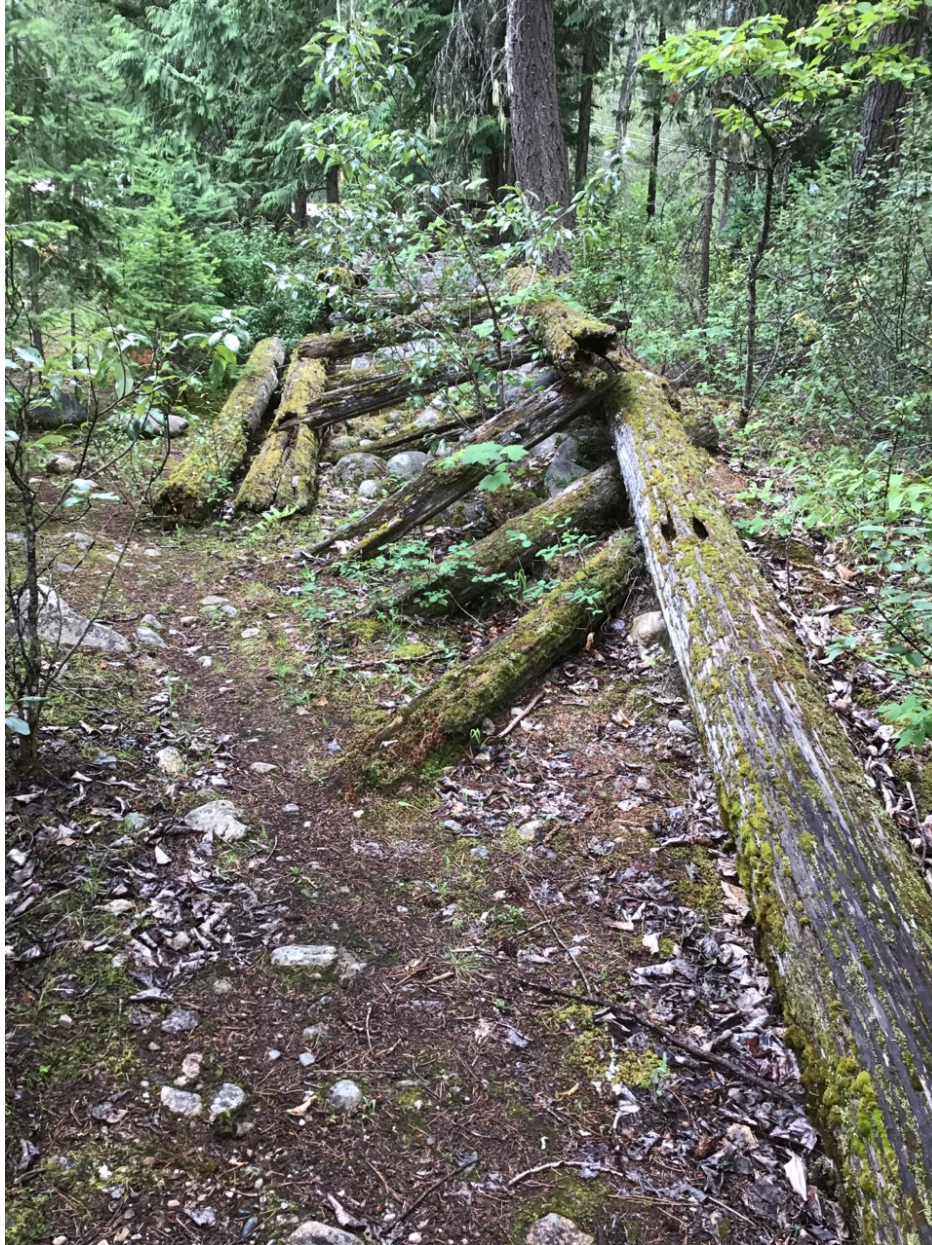
Figure 3-4. Failed log cribbing with gravel and cobbles along left bank of Lemon Creek. Photo: BGC, July 2, 2019.
