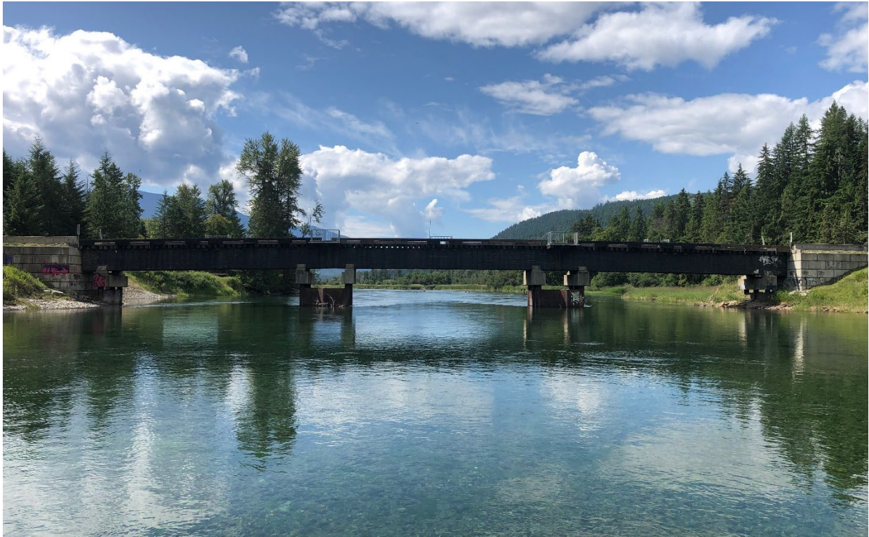
Figure E-13. Logging Road Bridge over the Slocan River looking downstream. Photo: Midwest Survey July 8, 2019.
