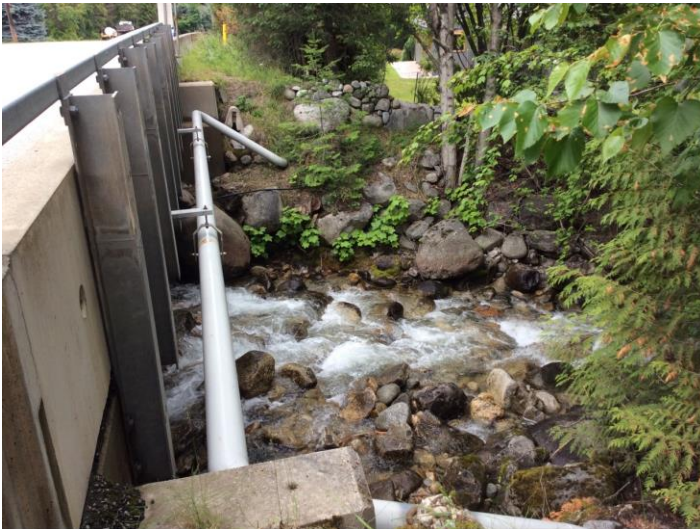
Photo 14. Standing on the right bank of Sitkum Creek downstream of the Highway bridge looking across at the left bank. Photo: BGC, July 4, 2019.
