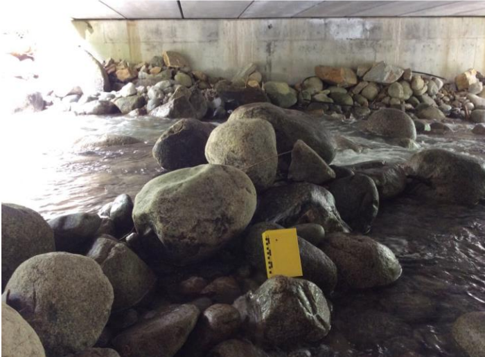
Photo 13. Underneath the highway bridge showing clearance as well as grain size (with notebook for scale). Photo: BGC, July 4, 2019.
