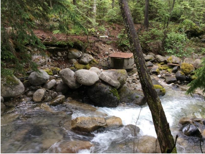
Photo 10. On right bank looking downstream at water intake, approximately 170 m upstream of the Hwy 3A bridge. Photo: BGC, July 4, 2019.
