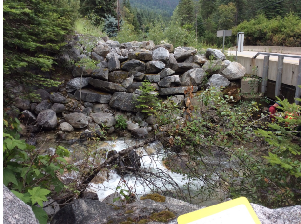
B) On right bank looking at left bank rip rap armouring approximately 1.5 m wide, 4 m high.
