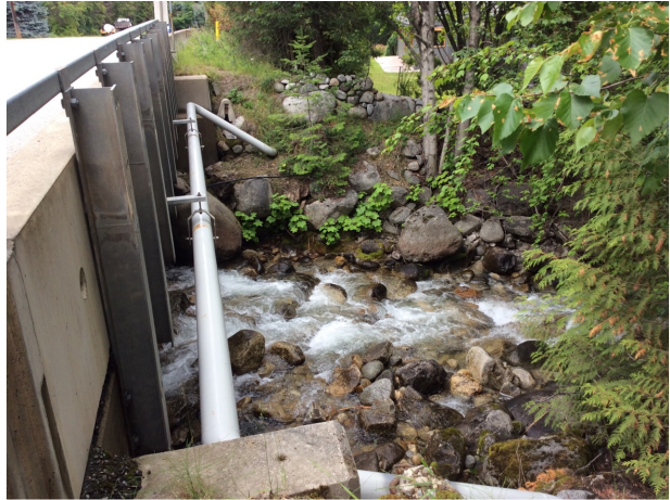
D) On right bank looking northeast at gas pipeline on downstream side of bridge.
