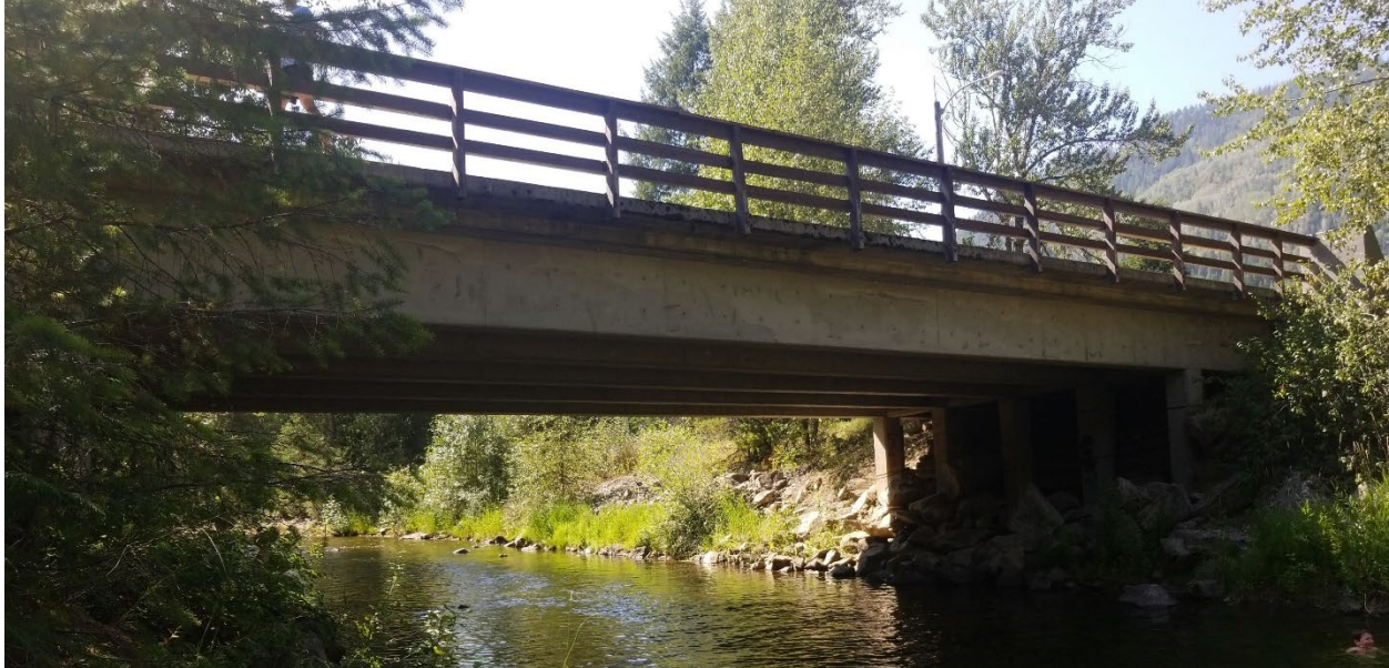
Figure E-19. Glendale Avenue / Main Street bridge over Erie Creek looking upstream (west) from the left bank. Photo: Midwest Survey August 6, 2019.
