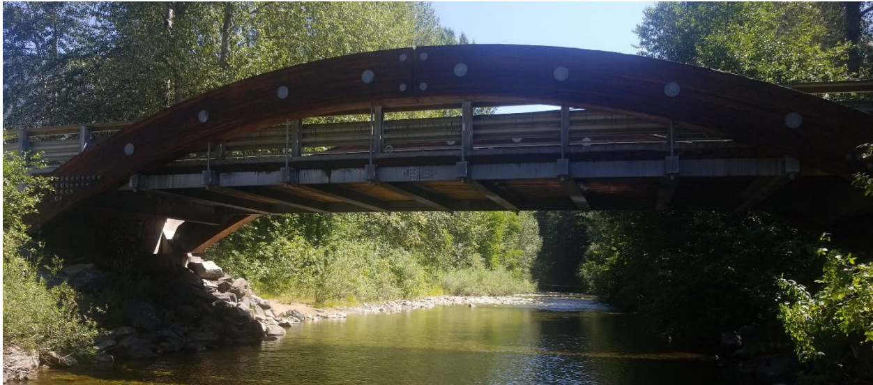
Figure E-17. Carney Bridge Road / Davies Avenue bridge over Erie Creek looking downstream (east). Photo: Midwest Survey August 8, 2019.
