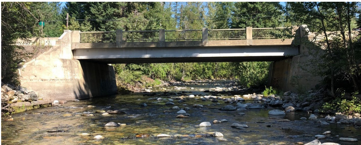
Figure E-14. Highway 3 bridge (upstream) over Erie Creek looking upstream (north). Photo: Midwest Survey August 7, 2019.
