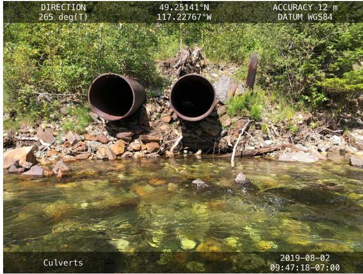
Photo 7. Culverts emptying into the Salmo River, approximately 2.5 km downstream of Porcupine Bridge. Photo: MSI, August 2, 2019.
