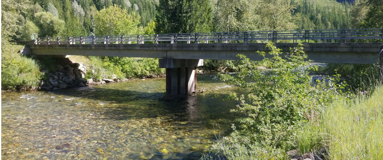
Figure E-9. Porcupine Road bridge over the Salmo River looking downstream (southeast). Photo: Midwest Survey July 28, 2019.
