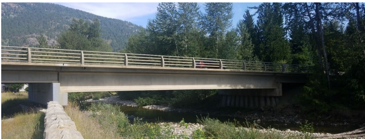
Figure E-16. Highway 3 bridge (downstream) over Erie Creek looking downstream (east) from the left bank. Photo: Midwest Survey August 8, 2019.
