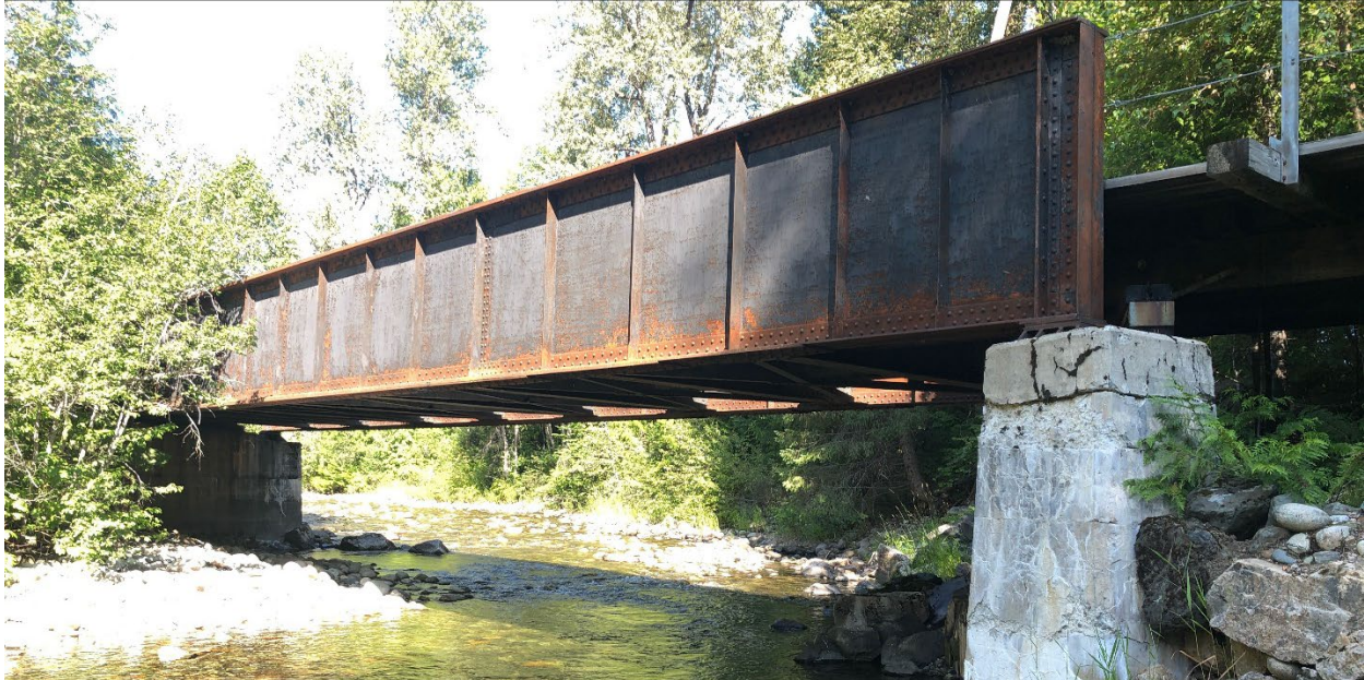
Figure E-15. Pedestrian bridge over Erie Creek looking upstream (northwest) from the right bank. Photo: Midwest Survey August 8, 2019.
