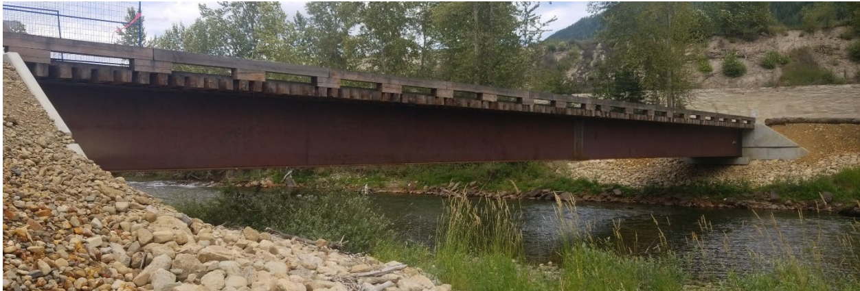
Figure E-13. Shambhala Grounds bridge over the Salmo River looking upstream (northeast) from the right bank. Photo: Midwest Survey July 29, 2019.
