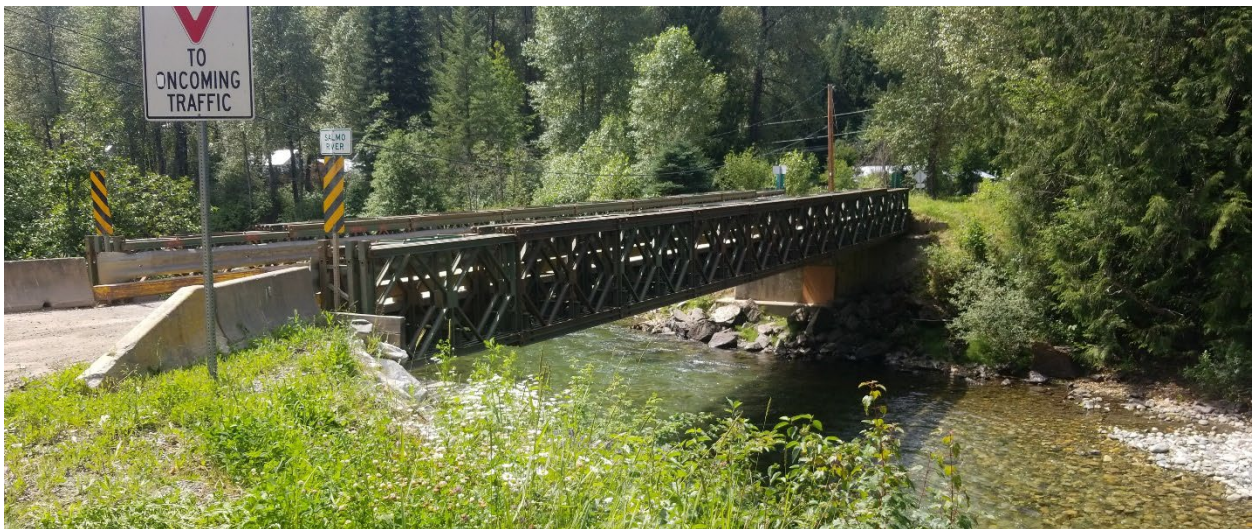
Figure E-8. Wildhorse Creek Road bridge over the Salmo River looking downstream (south). Photo: Midwest Survey July 28, 2019.
