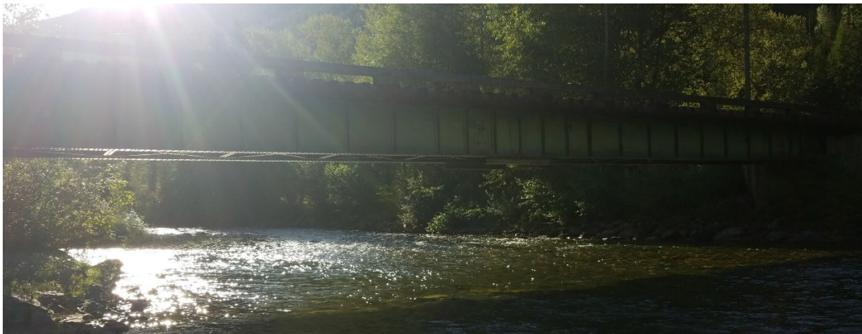
Figure E-10. Boulder Pit Road bridge over the Salmo River looking upstream (east). Photo: Midwest Survey July 29, 2019.
