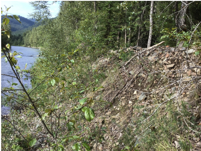
Photo 2. Dike steepened by erosion along the west bank of the Salmo River, approximately 800 m downstream of the confluence of Erie Creek. Photo: BGC, July 5, 2019.
