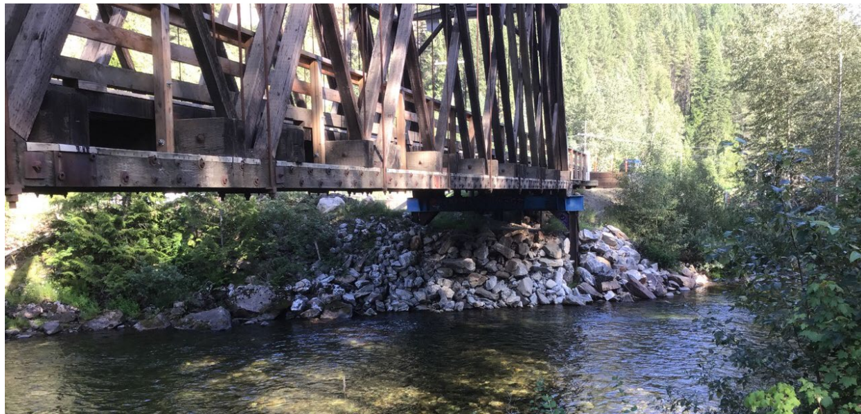
Figure E-11. Airport Road bridge over the Salmo River looking across (east) from the right bank. Photo: BGC Engineering July 31, 2019.
