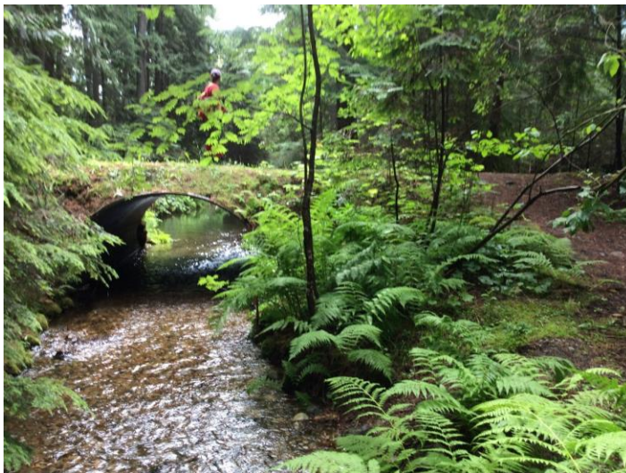
Photo 12. Standing approximately 120 m downstream of the gate shown in photo above and looking downstream, along the Redfish Creek spawning channel crossing with arch culvert. The arch culvert is approximately 3 m wide with 1.5 m of clearance to the water at the time of photo. Photo: BGC, July 3, 2019.
