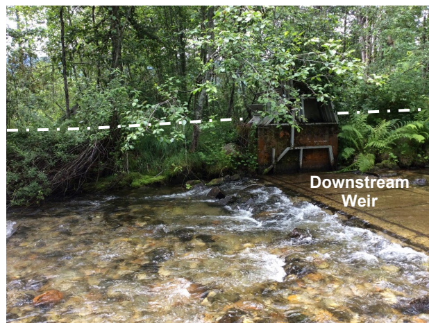
Looking southwest across creek at downstream weir, and Redfish Creek Dike (RFS-FP-03 located on the right bank). Dashed line indicates approximate dike crest.
