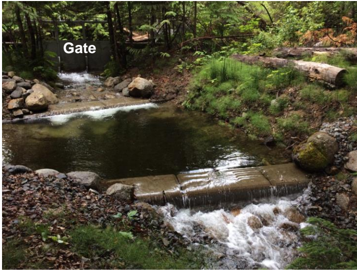
Photo 11. Looking upstream (north) at gate regulating flows diverted from Redfish Creek. In the foreground of the photo is the uppermost pool of the Redfish Creek spawning channel, partially built with prefabricated concrete blocks. Photo: BGC, July 3, 2019.
