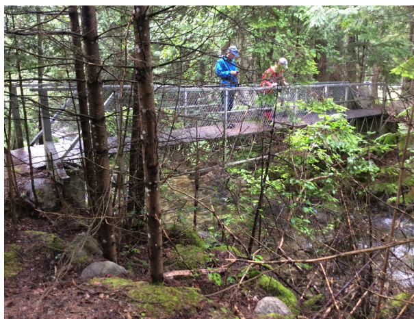
Standing on left bank looking south at the Footbridge. Creek flows from right to left in photo.
