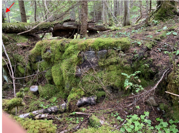
RFS-LP-02. Looking south at headwall of the old water intake on the right bank. For reference, note arrow indicating same tree as in image below.
