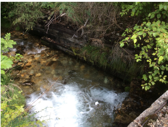
E) Looking downstream at outlet of railway culvert showing log crib bank protection.
