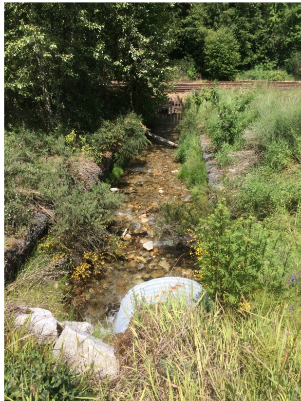
D) Looking downstream at gabion baskets lining creek from outlet of Railway Avenue towards railway.
