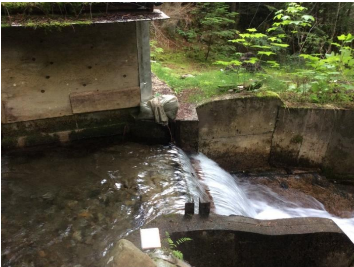
Photo 10. Looking downstream (north) at the water intake weir on Procter Creek. Photo: BGC, July 6, 2019.
