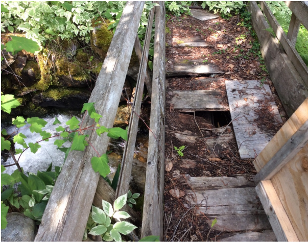
C) PRT-BR-3. Rotting footbridge over channel. Bridge is approximately 0.8 m high.
