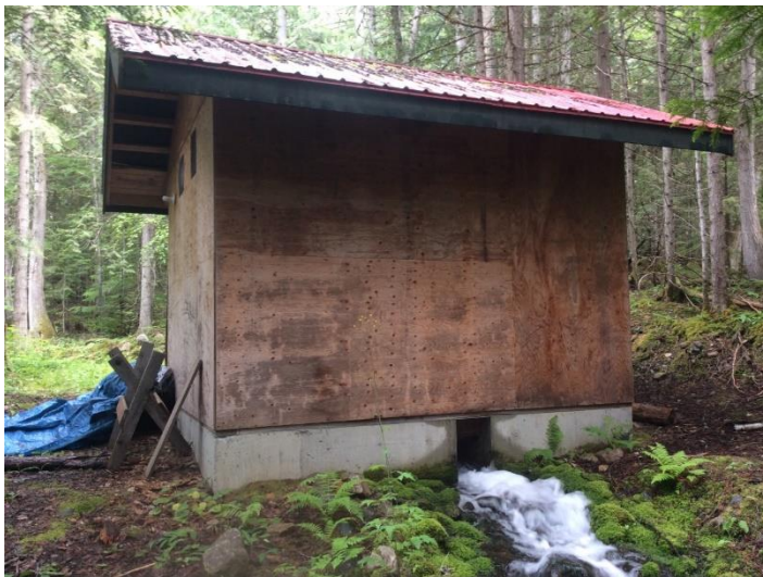
Photo 8. Powerhouse approximately 6 m east of channel, approximately 200 m downstream of the fan apex. Photo: BGC, July 6, 2019.
