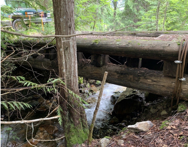
A) PRT-BR-1. Looking downstream towards wooden vehicle bridge approximately 130 m downstream of the fan apex.
