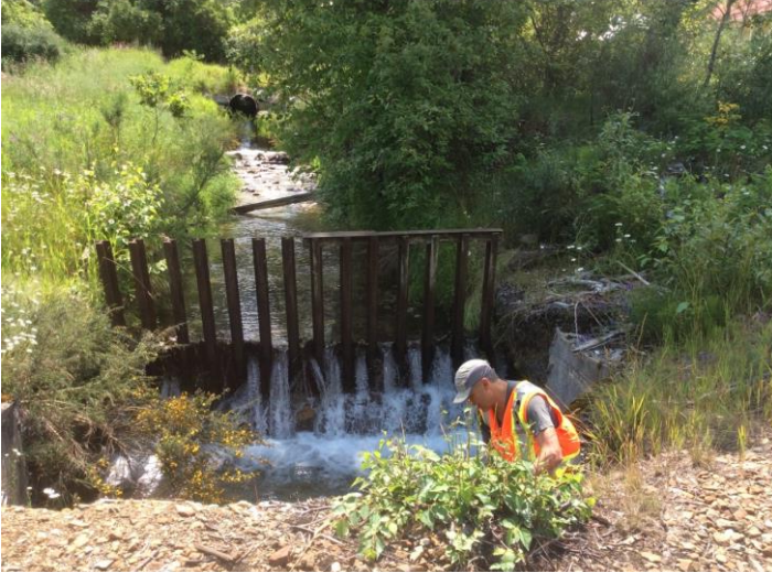
Photo 12. Looking upstream (south) at a trash rack made from cantilevered rails protecting the railway culverts. Photo: BGC, July 7, 2019.
