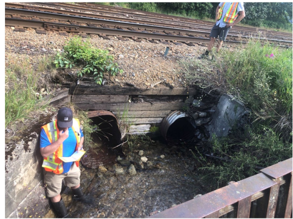
D) PRT-CV-4. Looking downstream at twin culverts under railway with trash rack in foreground.
