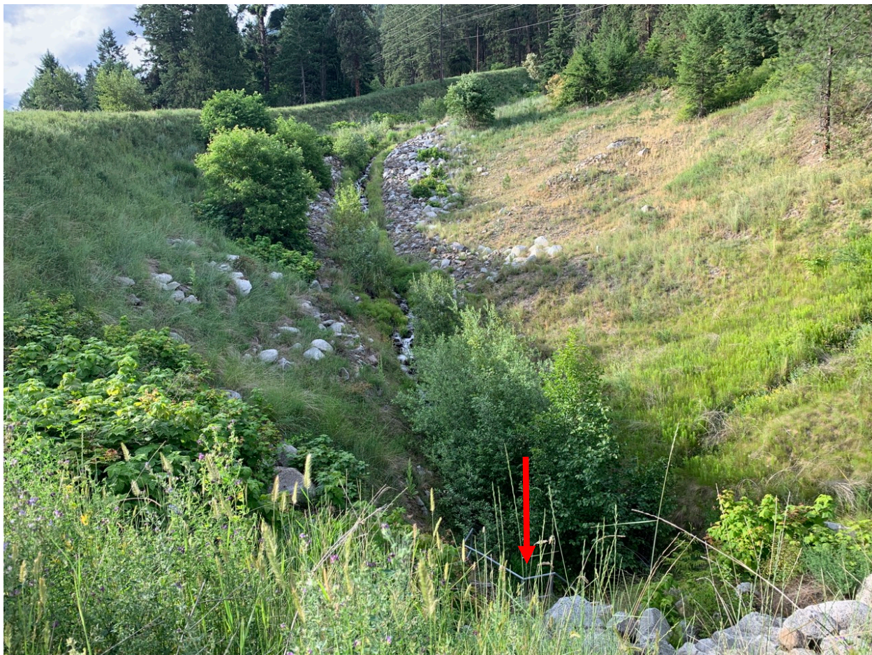
Figure 3-4. Location of debris basin culvert at downstream end of debris basin indicated by red arrow. Culvert inlet is constructed similarly to the spillway culvert shown in Figure 3-5 below. BGC photo taken July 10, 2019.
