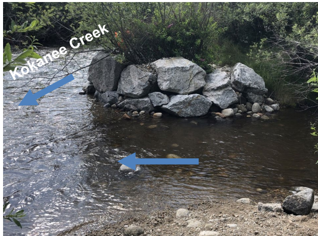
E) On the left bank of the Fish Spawning Channel outlet looking north at the end of KKN-FP-04 riprap.
