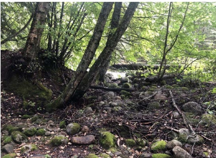
Photo 12. Standing approximately 50 m downstream of the footbridge looking at a failed dike. Photo: BGC, July 24, 2019.
