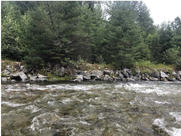
Photo 14. Standing on the right bank bar looking across (flow is left to right) at the cobble bar and flood protection on the right bank of Kokanee Creek, approximately 800 m upstream of the creek's mouth. Photo: July 24, 2019.
