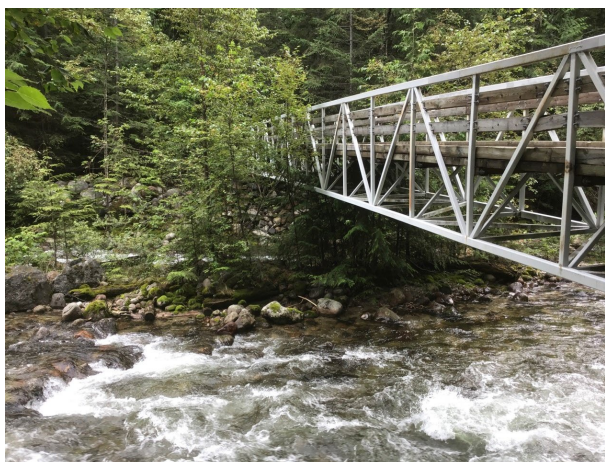
D) Standing on the upstream right bank looking at the upstream face of the Pedestrian Bridge.
