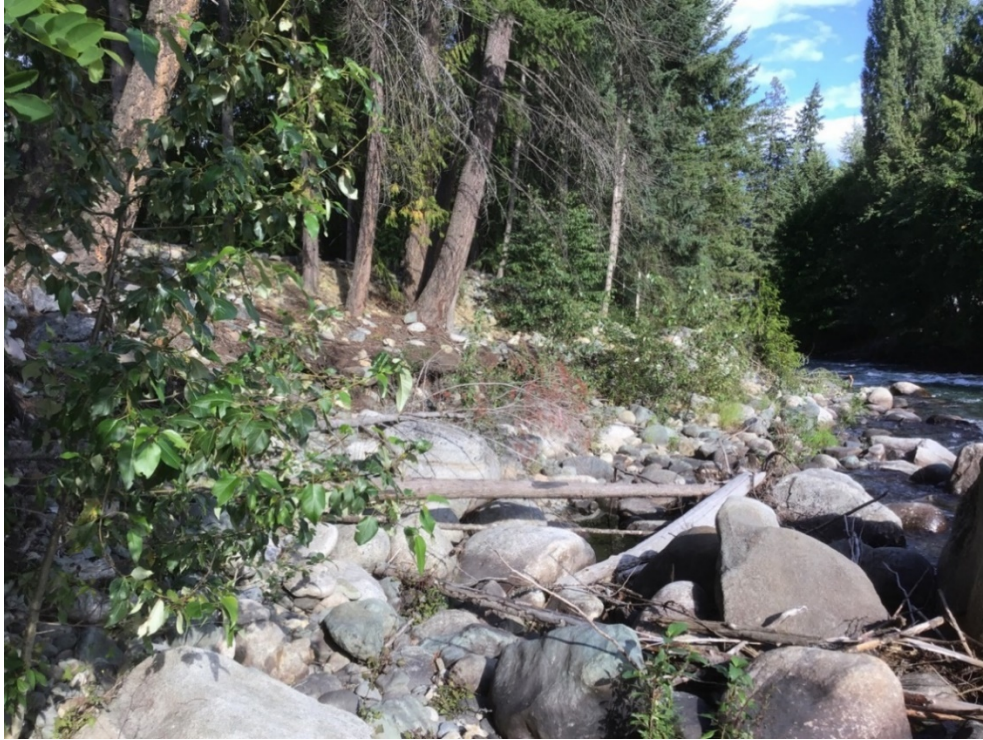
Figure 3-8. Tilted trees at the left (north bank) indicating bank instability processes (80 m upstream of the Highway 31 bridge).
