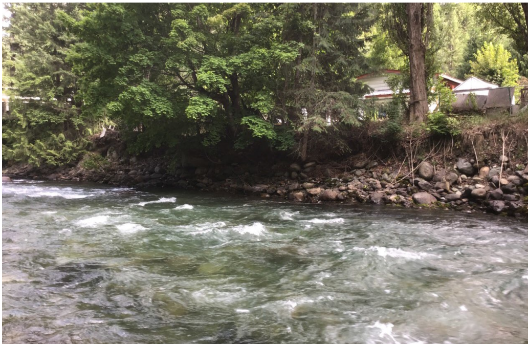
Figure 3-7. Bank erosion and slope instability upstream of the Highway 31 bridge (left bank). The depth of the undercutting is unknown, but local testimonials and previous reports suggest that it is a gradual process and has exacerbated for the past five years.
