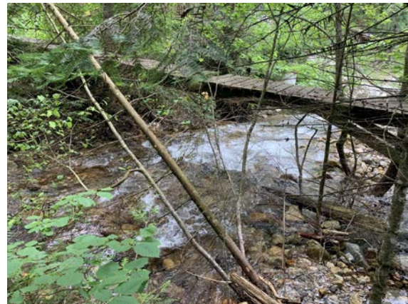
B) Wooden footbridge approximately 1.0 km upstream of Kootenay Lake. Condition is deteriorating.
