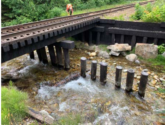
E) Standing on right bank looking west at railway bridge crossing Harrop Creek and log crib structure.
