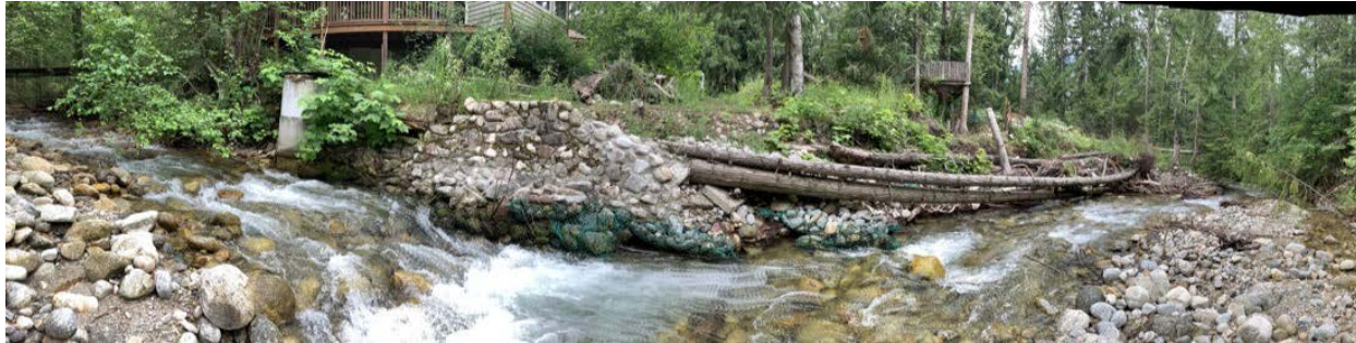
HRP-FP-04 – Bank erosion on outer (left) bank approximately 2 m tall. Note; house in the background, makeshift erosion protection with cemented stone wall on top deformed, green wire-mesh baskets, and logs placed further downstream.
