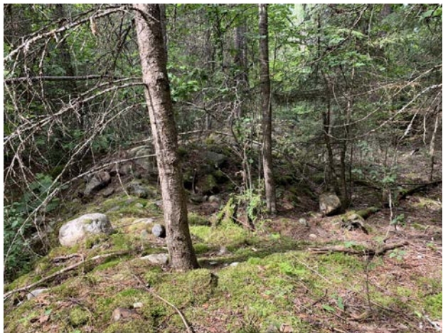
HRP-FP-05 – Non-engineered dike on right bank made from rounded river rock.
