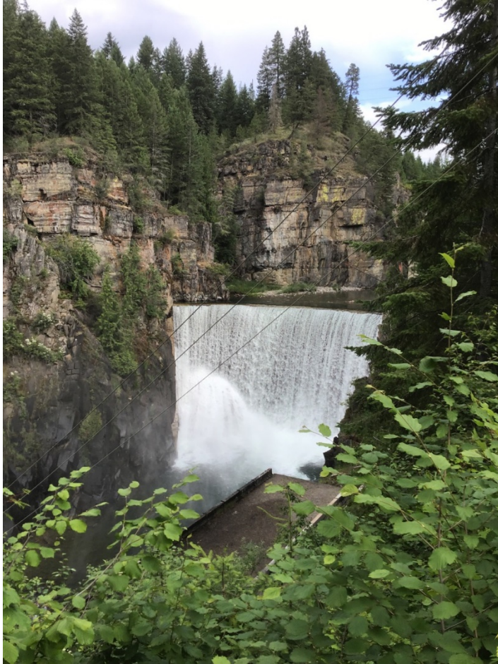
Photo 1. Goat River Dam, approximately 11 km upstream of the outlet to Kootenay River, looking upstream (northwest). Photo: BGC, July 16, 2019.
