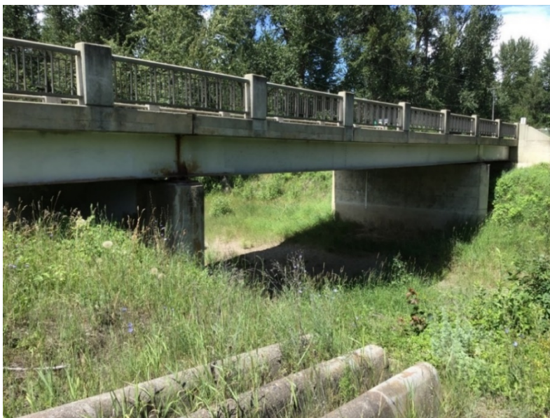
Figure 3-6. View from upstream of the Highway 21 bridge looking downstream (west) at the dry secondary (south) channel of the Goat River. Photo: BGC, July 3, 2019.
