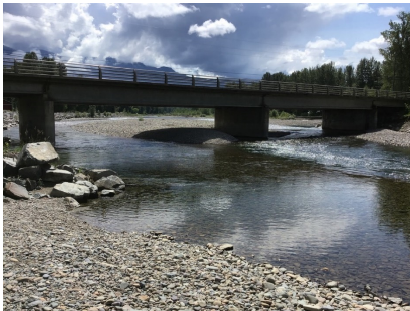
Figure 3-5. View from downstream of the Highway 21 bridge over the main (north) channel of the Goat River looking upstream (east). Photo: BGC, July 3, 2019.
