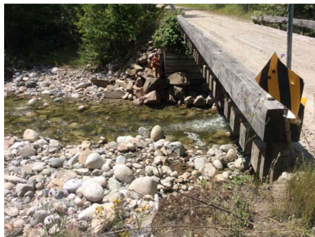
B) EGL-BR-1. Standing on right bank looking at left bank retaining wall and rip rap.
