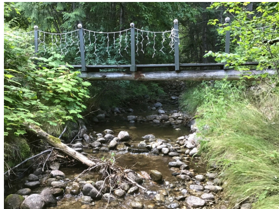
F) Pedestrian Bridge 2, approximately 70 m downstream of Lower 6 Mile Road East Bridge.
