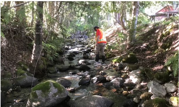
C) DHL-FP-10 & 11: Approximately 110 m downstream of bifurcation looking upstream. Minimal protection on either bank
