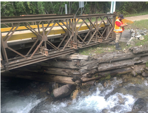
C) Looking at the right bank (west) at the DHL-FP-02 and Duhamel Creek Rd Bridge on the left.
