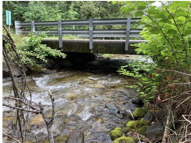
D) Looking downstream at Lower 6 Mile Road West Bridge over western channel.
