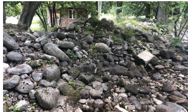
D) DHL-FP-06: Berm constructed of sub-rounded cobbles and old concrete foundation approximately 40 m upstream left bank of Lower 6 Mile Road on the western channel.
