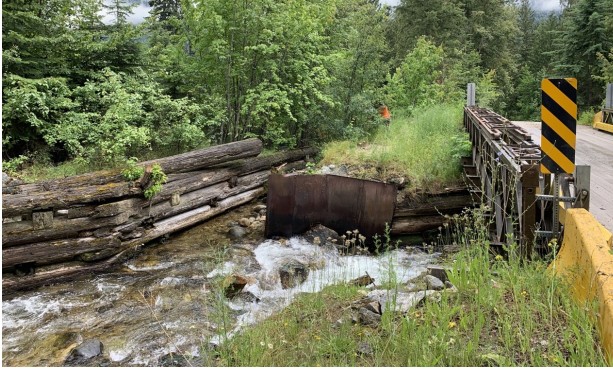
A) Looking downstream (south) at DHL-FP-01 (on the left) and DHL-FP-03 (bifurcation structure "V") with Duhamel Creek Road Bridge on the right.
