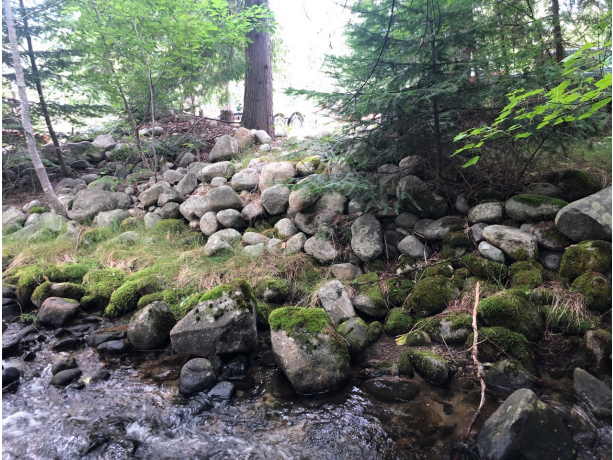
A) DHL-FP-12: In the channel looking at left bank immediately downstream of Highway 3A.
