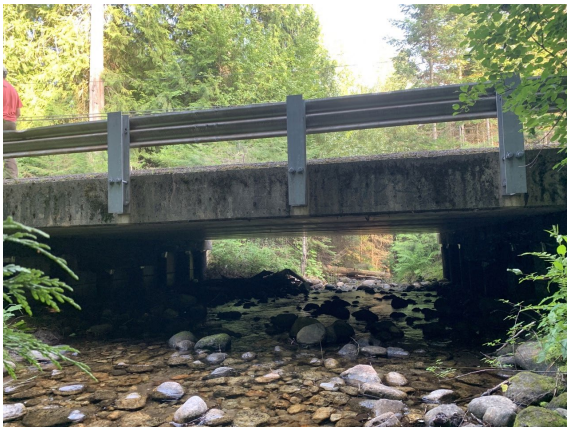
E) Looking downstream at the clearance of the Lower 6 Mile Road East Bridge across the eastern channel.
