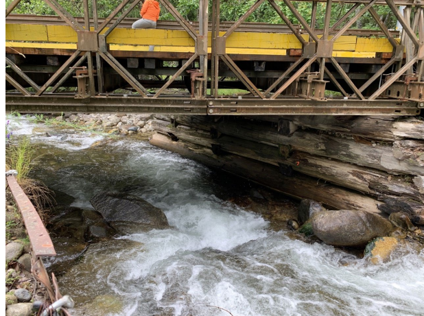
B) Looking downstream (towards western channel) underneath Bifurcation Bridge at the bifurcation structure (see also Photos 4 and 5 in Appendix B for aerial view of bridge).
