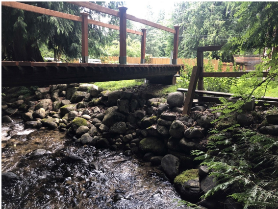
C) Looking downstream at Pedestrian Bridge 1 approximately 50 m downstream of Duhamel Highway 3A East Bridge on the eastern channel.
