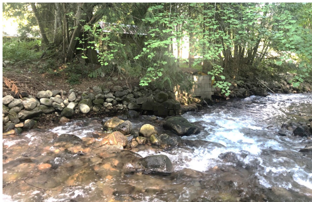
D) DHL-FP-04: Placed creek bed material on left bank approximately 130 m upstream of Highway 3A. Concrete brick wall and water intake visible in the distance
