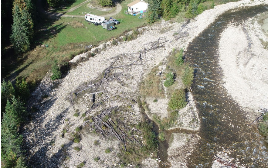
Photo 19. Drone Photo of Dyke along Crawford Creek's west bank, 450m north of Highway 3A. Photo: Explore, September 25, 2019.
