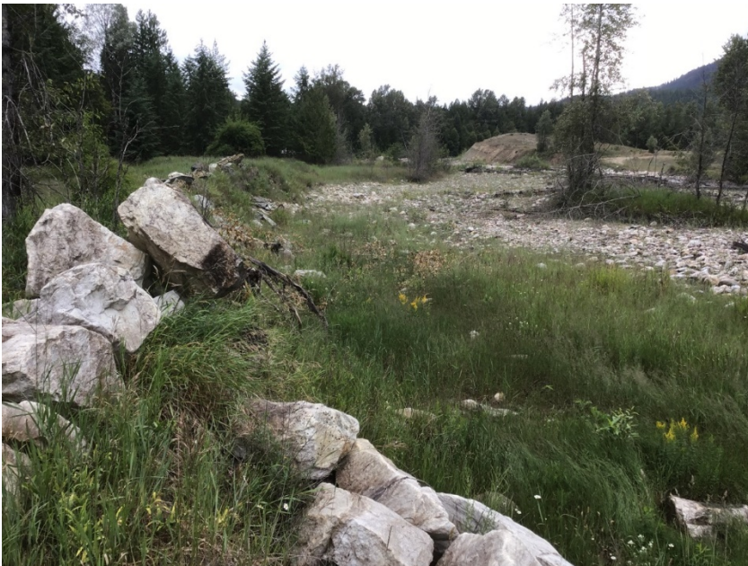
Photo 16. Bank protection along Crawford Creek's west bank, 360m north of the Highway 3A. Photo: BGC, July 4, 2019.
