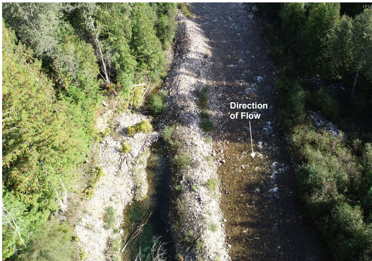
Figure 3-6. Overgrown section of dike along Crawford Creek's west bank, 600 m north of the Highway 3A. Photo: Explore, September 25, 2019.
