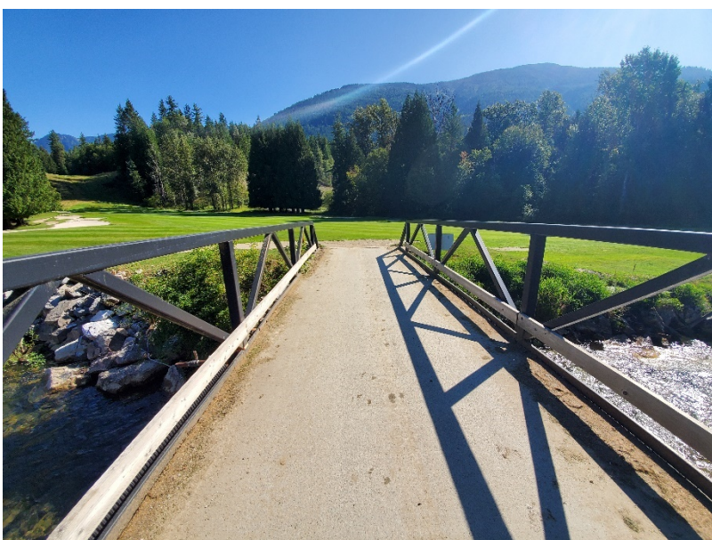
Photo 11. Pedestrian Bridge crossing Crawford Creek, 200 m north of Highway 3A looking to left bank. Photo: Explore, August 28, 2019.
