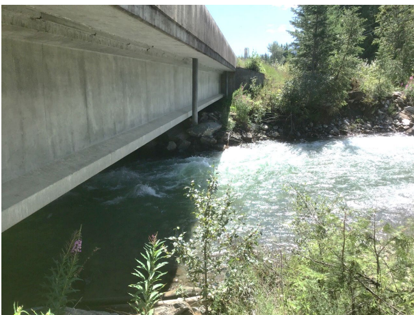
E) Looking at Cooper Highway Bridge from the left (north) bank on upstream side.
