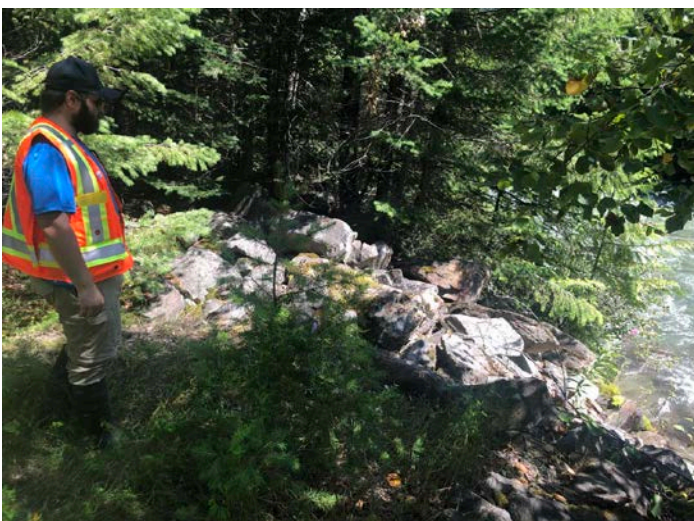
Photo 14. Standing immediately downstream of the Highway 31 bridge on the left (north) bank looking at the riprap. Photo: BGC, July 25, 2019.
