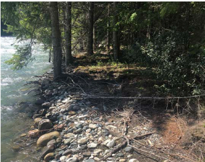
Photo 16. Standing on the left (north) bank of Cooper Creek looking upstream at bank erosion, approximately 200 m downstream of the Cooper Creek Highway bridge. Photo: BGC, July 25, 2019.
