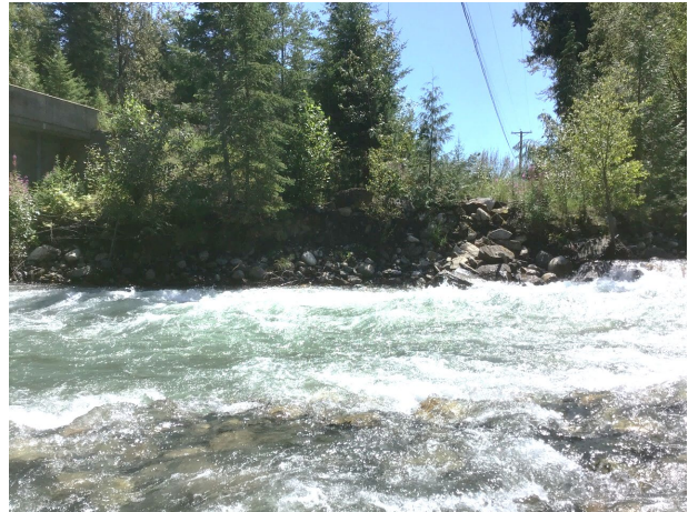
D) On upstream left bank looking across at riprap on right bank, upstream of Cooper Highway Bridge.
