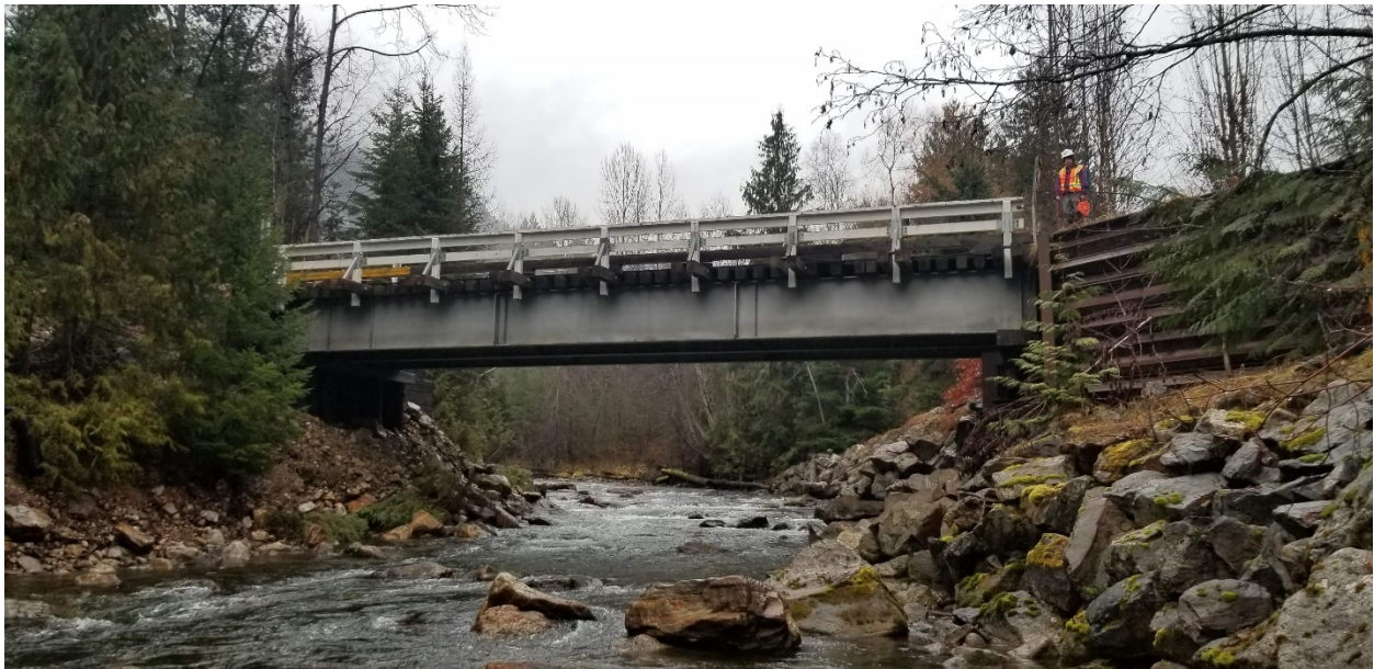
Figure 3-6. View from downstream of the McCormack Road bridge on Caribou Creek. Photo: BGC, November 22, 2019.
