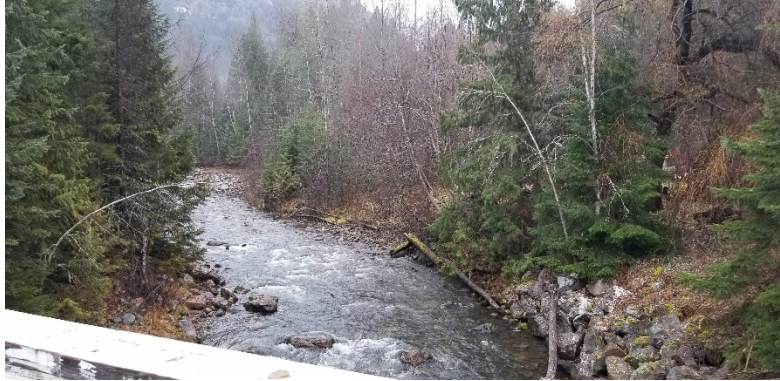
Photo 9. Looking upstream from the McCormack Road bridge looking east showing placed riprap along left bank. Photo: BGC, November 22, 2019.
