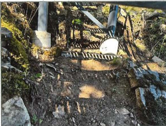
Photo 9. Disturbed soil under stairway
