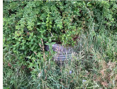
Surface Water Cannot Flow In
