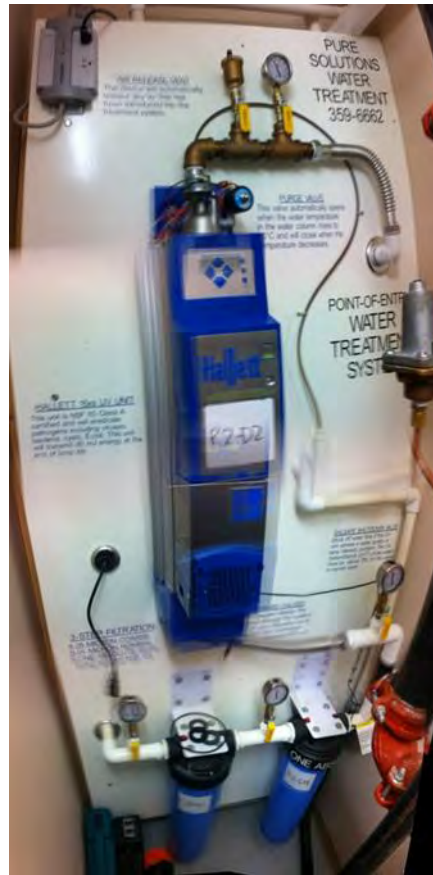
Figure 9: Point of Entry Treatment System
