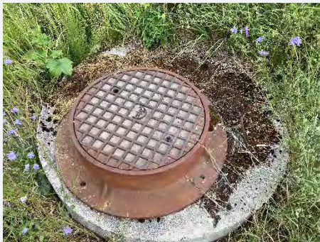
Unsecured Cover – No Grate
