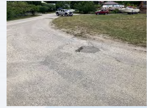
No Catch Basin at Tee
