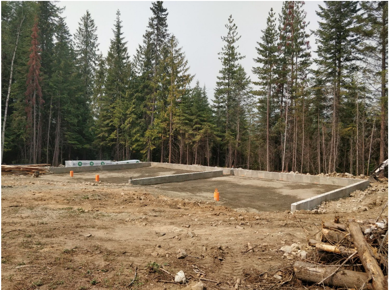
Figure 6 - Partially constructed storage building that has been constructed prior to issuance of building permit.
